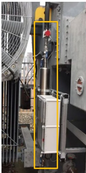
Fitted to a 30 MVA
