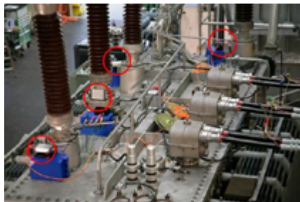
Fig. 7 PD measurement on a 110kV transformer
