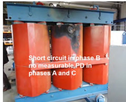
Fig. 10 Breakdown fault on a transformer
