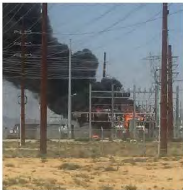
Image #1: Transformer Failure
