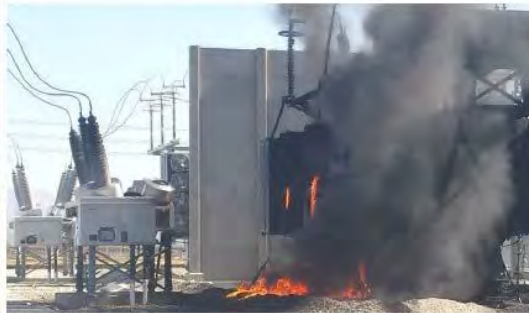
Image #2: Transformer Failure
