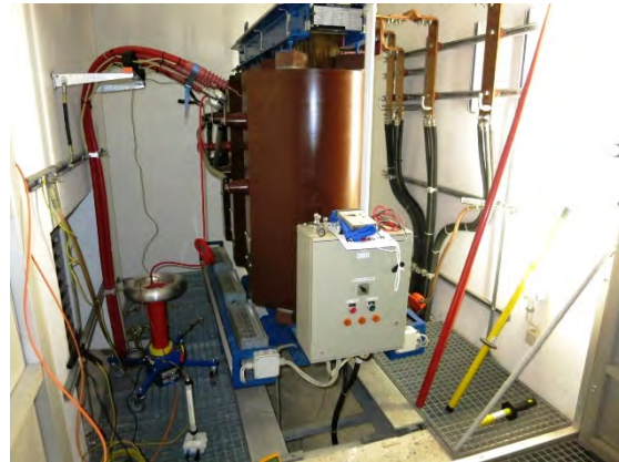
Fig. 14 PD measurement setup on a 20kV / 2MVA transformer
