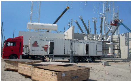
Fig. 13: On-site PD testing on 500MVA current limiting reactors
