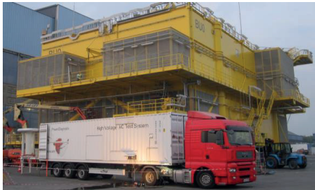
Fig. 1: Inverter based AC mobile test system
