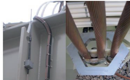
Fig. 16: Left, a disturbance antenna under an open air bushing, Right, a HFCT in the ground loop
