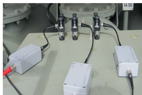
Fig 20: Acoustic sensors fitted with magnetic holders to a transformer oil bushing
