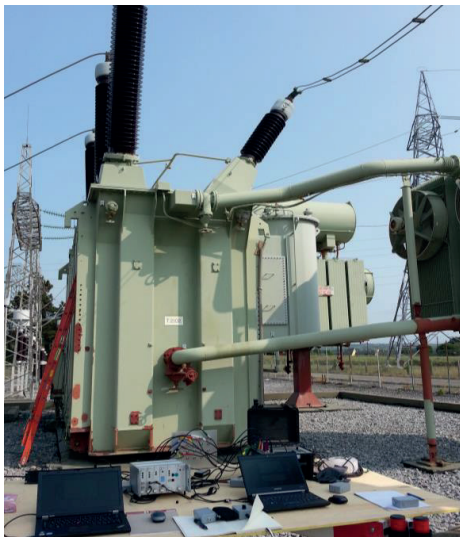
Fig. 3: On-site partial discharge measurements
