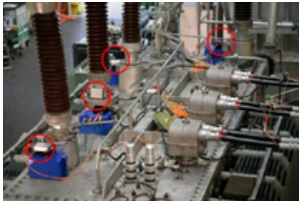
Fig. 7 PD measurement on a 110kV transformer
