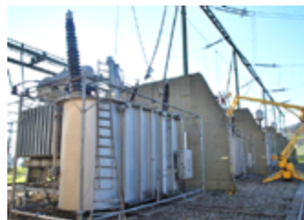
Figure 8: 220/150 kV, 140 MVA single phase transformer
