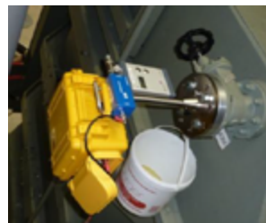
Fig. 22 UHF sensor mounted on the main drain valve
