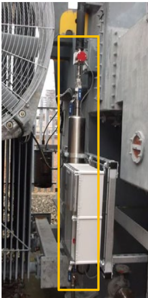
Fitted to a 30 MVA
