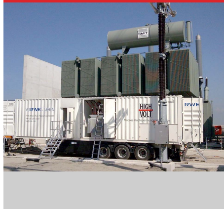
On-site test systems
