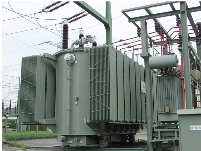
Figure 2: Hermetically sealed transformer
