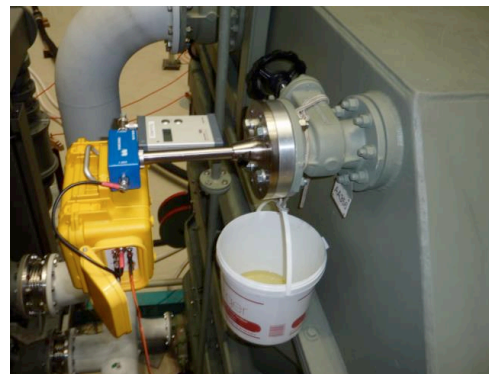
Figure 4: Installed UHF probe
