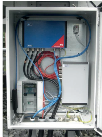
Fig. 28 Bushing monitoring system MONTRANO
