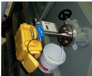
Fig. 23 UHF sensor mounted on the main drain valve
